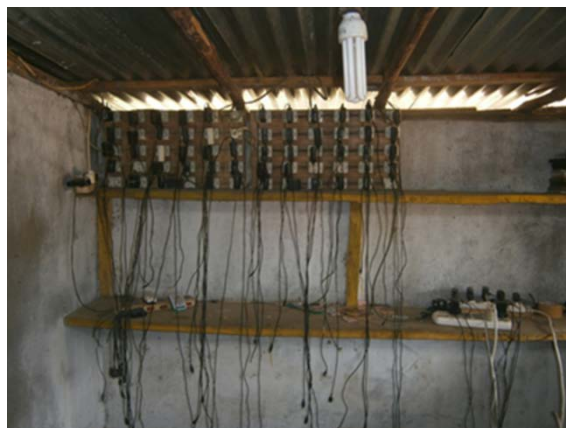
Figure 12 - (An empty) Charging station in Port Loko that had been shut down for three months due to generator failure
